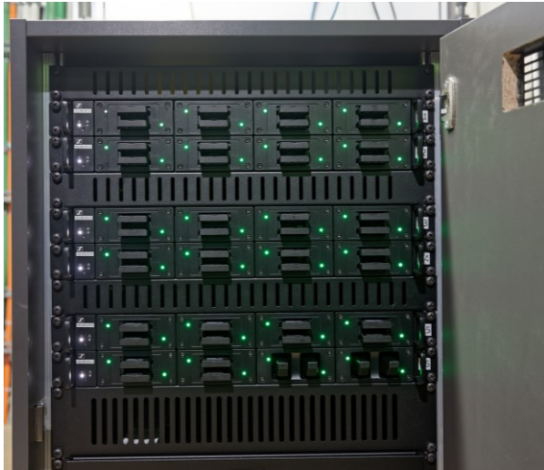
Six L 6000 charging stations provide power for the batteries
